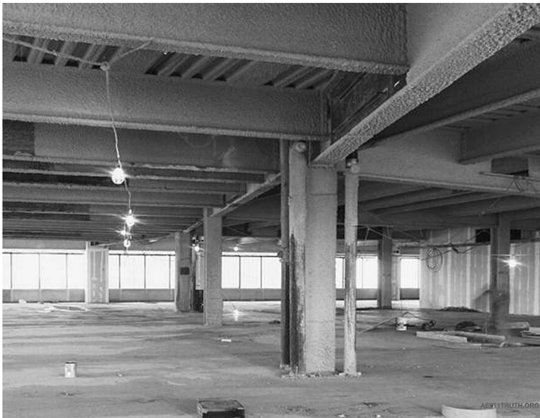
Figure 8. The vertical member in the center is World Trade Center Building 7's column #79. The larger horizontal beams that are directly connected to it are the girders, and the horizontal beams that are connected to the girders are the floor beams.
