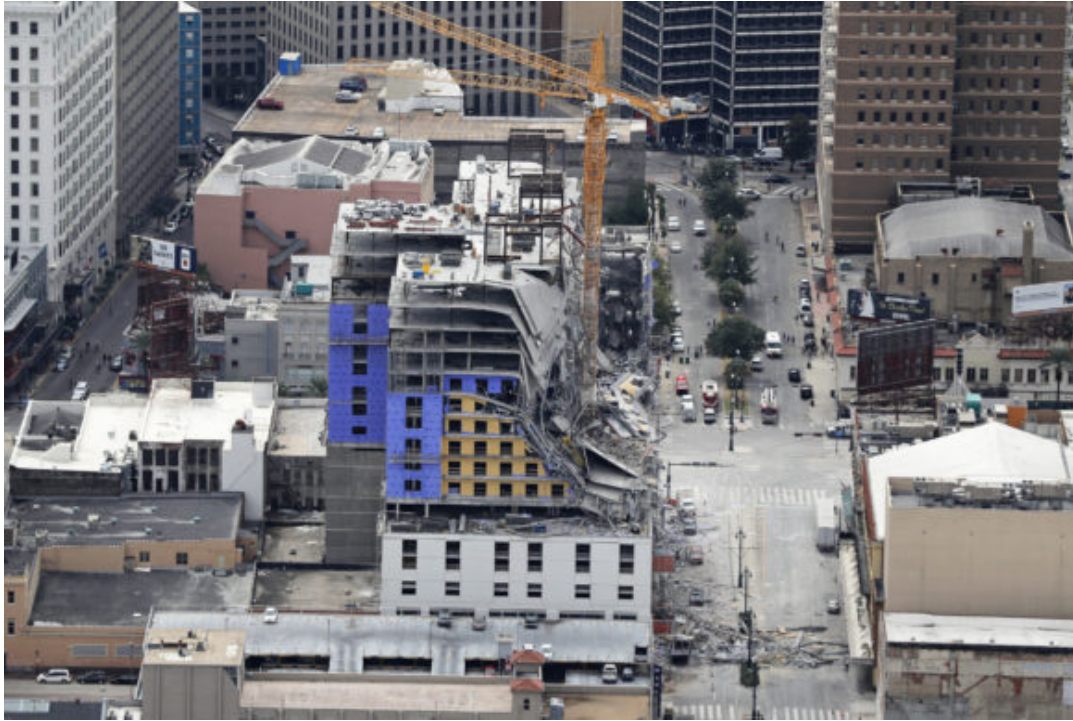
This building is missing a column or two. It didn't collapse
